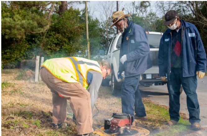
SC Rural Water Infrastructure Authority and Richland County Utilities Department working with Town of Eastover employees on installing smoke test device. Photo by Michael Dantzler
