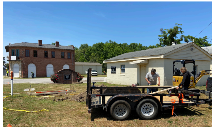
Construction has started on the Town's marquee that should be completed in a few weeks. Photo by Michael Dantzler
